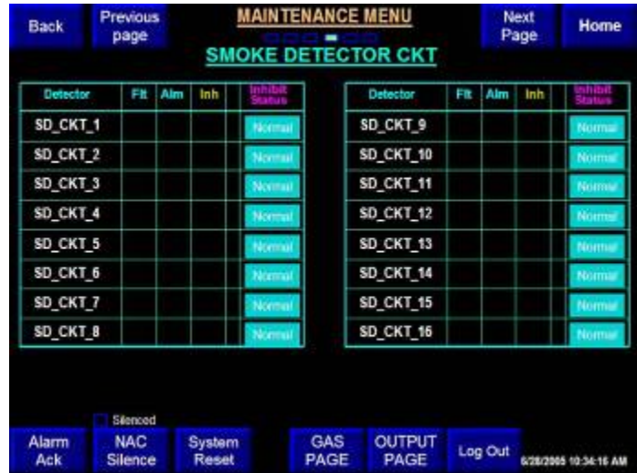
Figure 10: Fire Alarm Maintenance Screen
